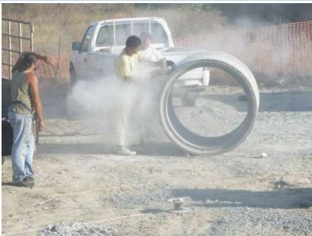
Complete lack of use of PPE during the use of a cement cutter
