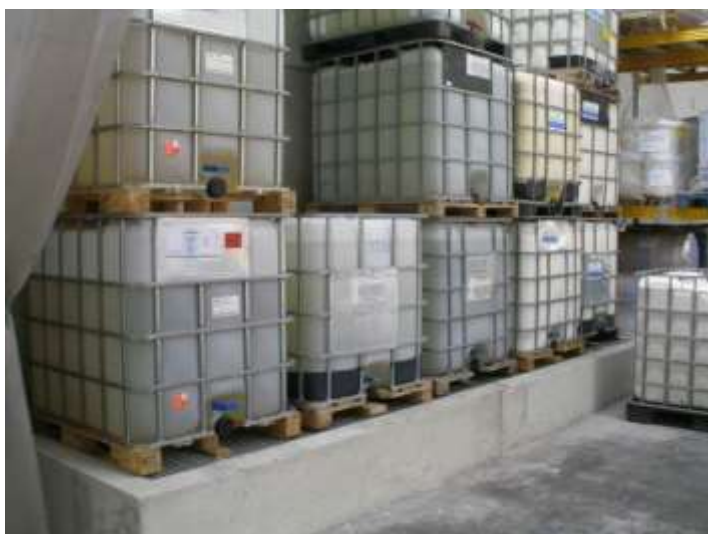
Secondary containment (dike) under IBC's.
